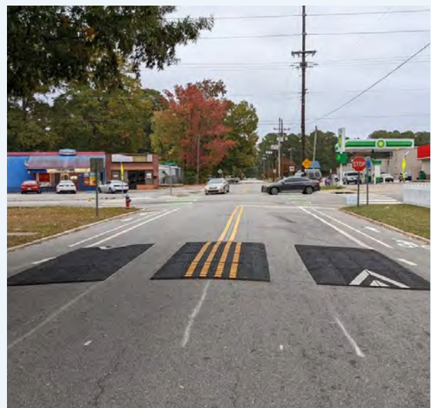
In the City of Rocky Mount, speed cushions have been implemented to strategically calm traffic.
